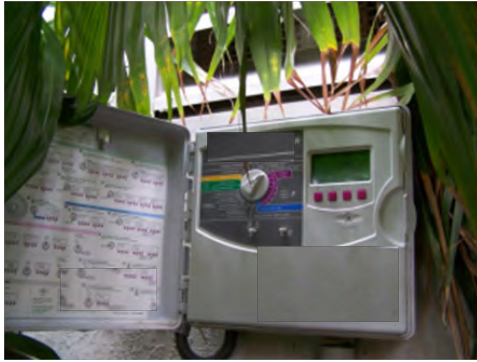
Figure 55. A smart irrigation system control box.
