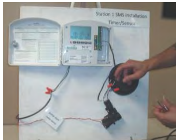
Figure 54. A demonstration of proper wiring of a soil moisture sensor.
