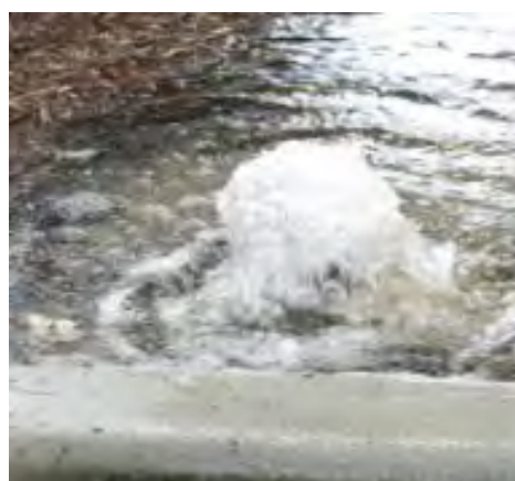
Figure 46. Broken sprinkler head creating a “geyser.”
