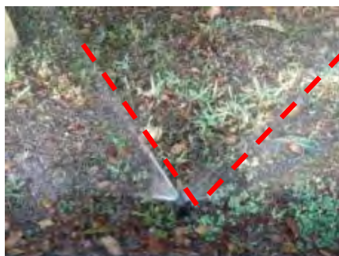
Figure 47. Clogged sprayhead, the area between the two dashed red lines is not receiving water.
